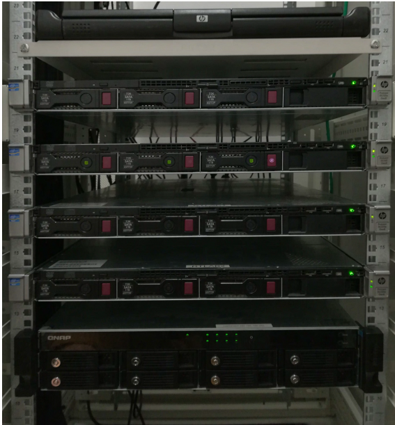
FIGURE 10. Communications cabinet servers.
