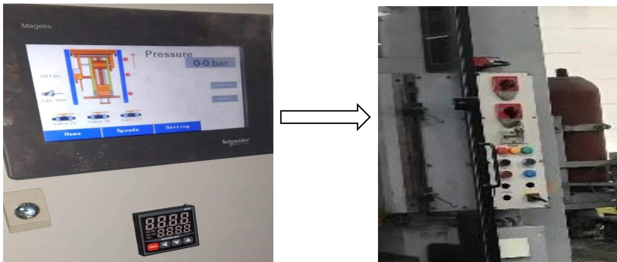
Fig. 3. Integrated HMI screen (left) and old control system (right)
