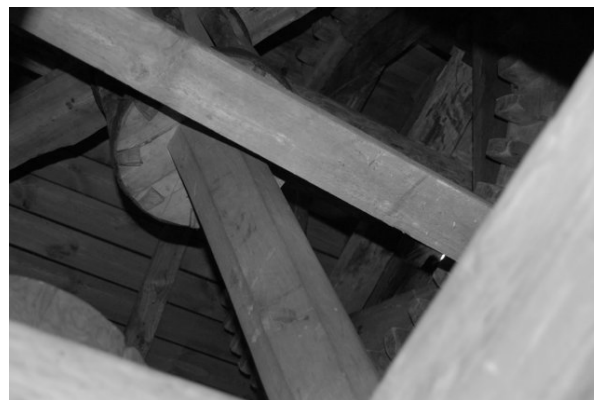
Figure 2: Old traditional gearbox opened for checking the wear of gear teeth
